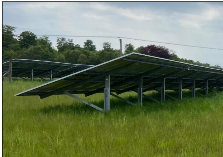
Figure 4: Example PV Mounting System 2 Single row of piled uprights penetrating the ground 2
