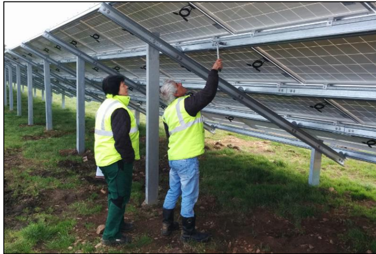
Figure 3: Example PV Ground Mounting System 1 Supporting pile uprights front and back 1
